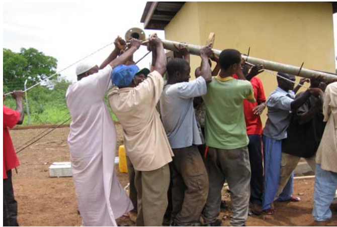
fig 1. Leaders and Youth of Bimbilla volunteer to help install repair the borehole
