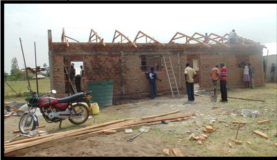
Building the roof of The Tumaini Learning and Development Center and adjacent Class 1 classroom
