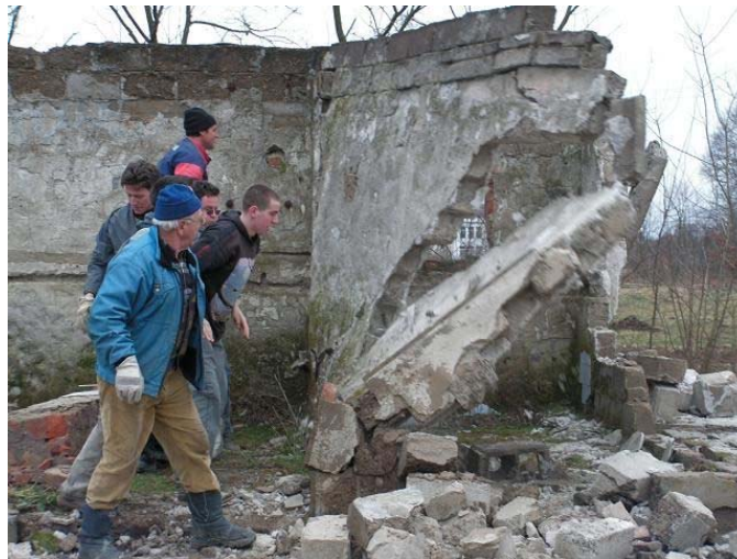
The community unites to bring down the old walls on July 22 nd , 2007
