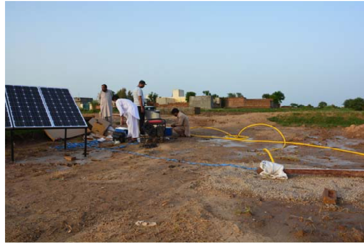
The blue power cords extend into the bore hole (marked by the white bag) while workers attend to the converter that transfers power from the solar collector into an electric current.
