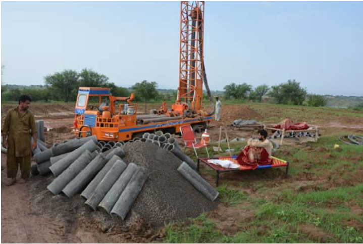
The drilling rig in place, with filter pipes waiting to be lowered. A drill worker rests on his bed, where he slept during the round-the-clock drilling process.
